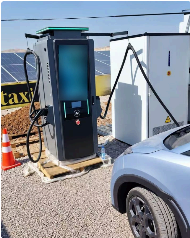
A DC fast charger beside an electric car, with two charging cables.
